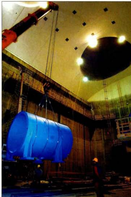
Inside the ATLAS cavern: manipulating shielding to fit within the beam tunnel.
